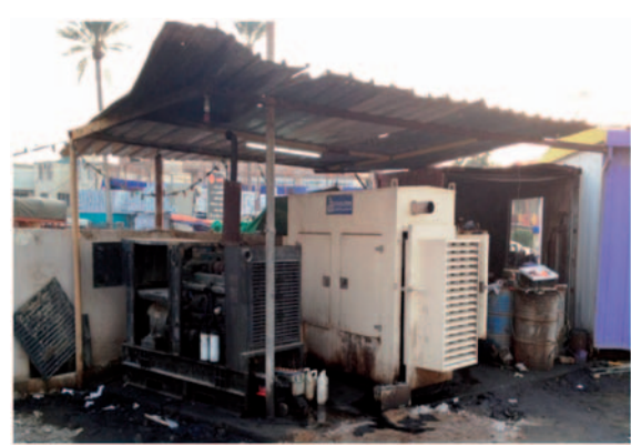
Figure 1. Generators are everywhere in Iraq: majority are run on a commercial basis at heavy costs to families and businesses (Courtesy: Rawaf 11 ).
